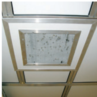
Shielded air vent
